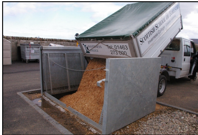
Figure 3.2: Below ground wood chip storage at Inverness College. (Photo courtesy of Highland Wood Energy)
