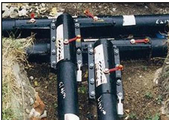
Figure 3.3: Pre-insulated heat main (Source: Community Heating – a guide 4 )
